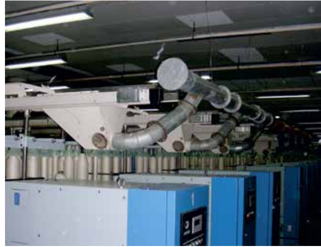
Fig. 13 - Discharge of the travelling blower
