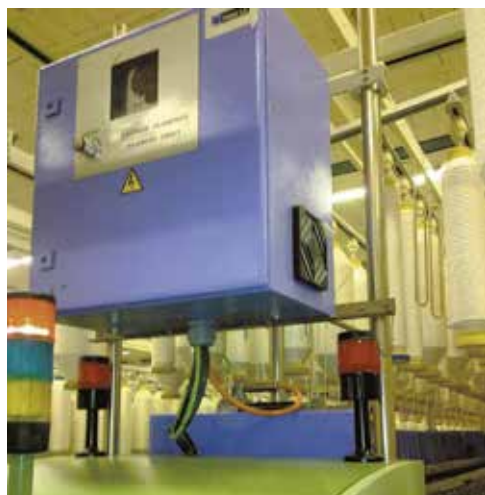
Fig. 14 - Other special drives in the area of the creel
